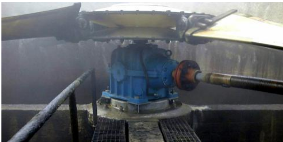
Gearboxes TSA 031 351-07, power station Tisová, Czech Republic
