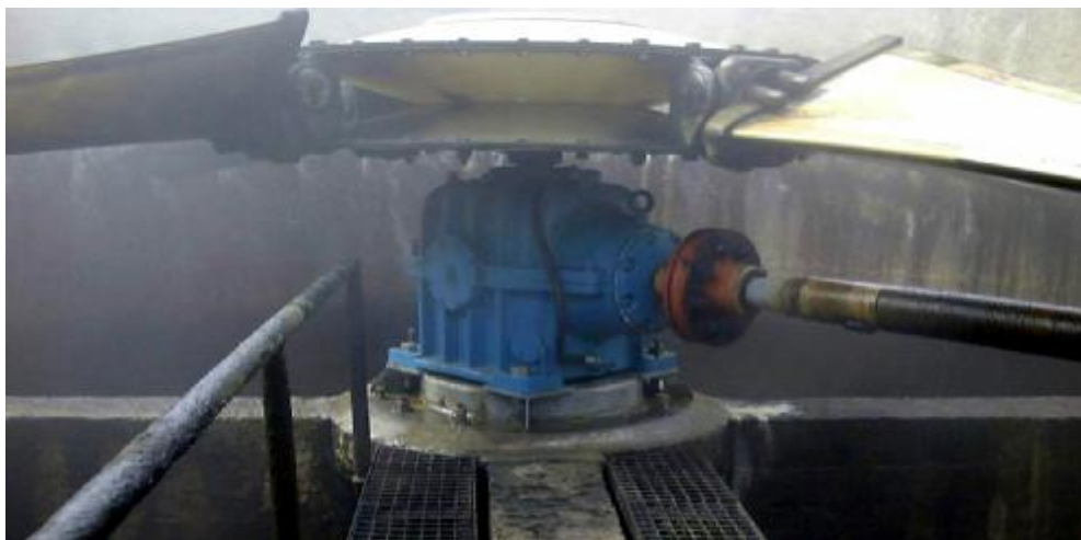
Gearboxes TSA 031 351-07, power station Tisová, Czech Republic
